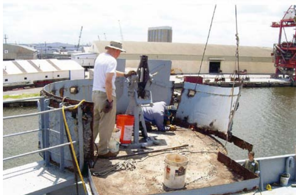
Chief Mate Larry Knapp, at the 20 mm gun mount, watches as Bob Jackson uses a cutting torch to remove a section of the starboard gun tub. Visible at lower right is Bien Gamboa serving as the fire watch. The piece being cut is held by a wire sling connected to the ship's cargo gear at hatch #1.
