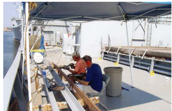
Volunteers Gary Eng and Don Webster use needle guns on the heavy angled pipe guards that protect the piping that runs alongside #2 hatch. The replaced steam line is the upper of the two pipe runs shown in the background running alongside #2 hatch.
